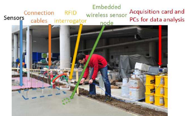
Figure 2 : Outdoor deployment of CNT sensors in Sense-City demonstrator
